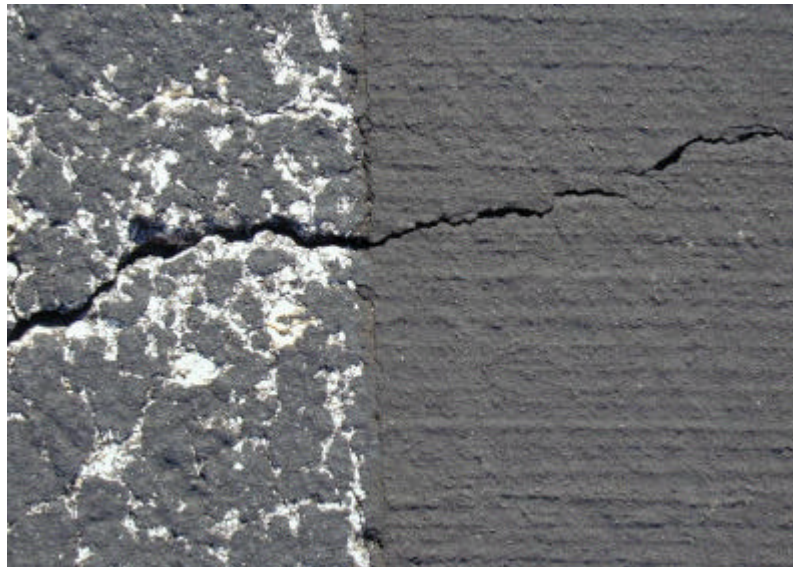
Figure 5. PCMO section at MacDill AFB showing reflective cracking. Note that the crack has not widened or displayed any raveling from the crack face.
