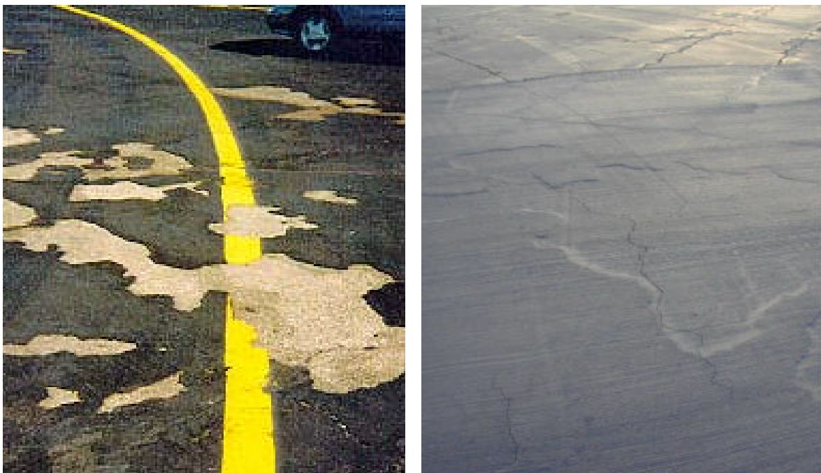
Figure 7. “Delaminated coal tar area before (1998) and after sealing with PCMO (2000) at Forbes Field, Topeka, KS.
